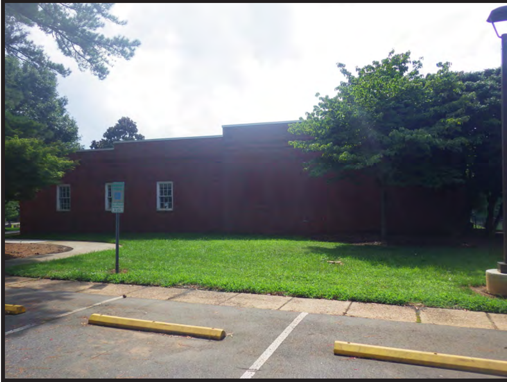
Figure 21. Agriculture Building, East Side with 1928 Section Right of Frame and Circa 1950 Section Left of Frame (With Windows)
